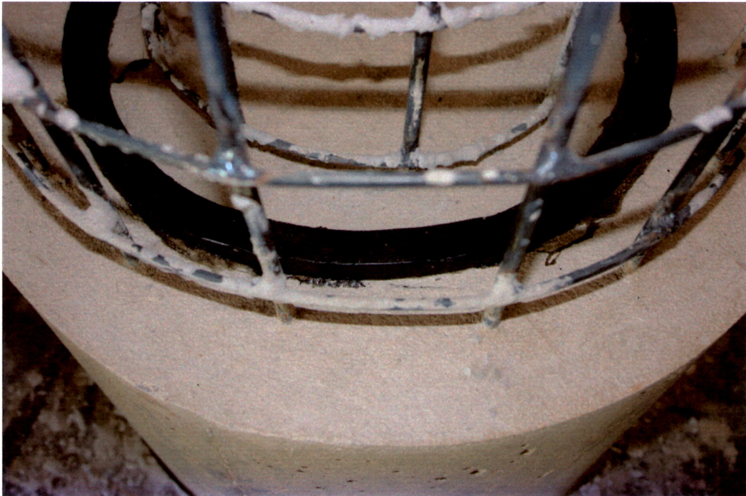
Photograph 1 - Bond Swelling installed along the construction joint of the concrete test chamber
